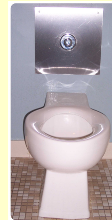
Concealed Toilet Plumbing
